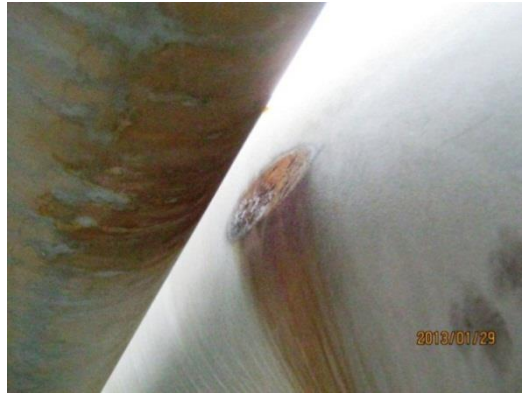
Figure2. The erosion of pipeline 16 inches on adjacent pipeline
