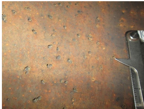
Figure6. The pitting on inner surface of straight stream of pipeline
