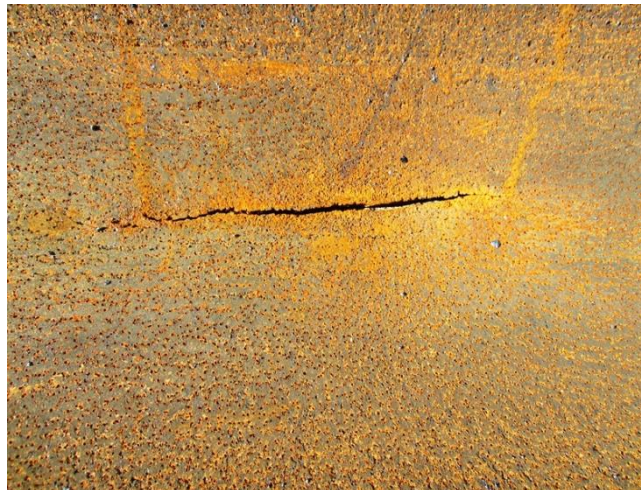
Figure4. Groove on the surface of pipeline
